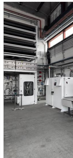
Onsite hydrogen production
