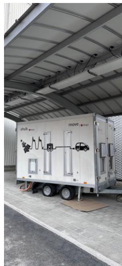
Battery buffer storage
